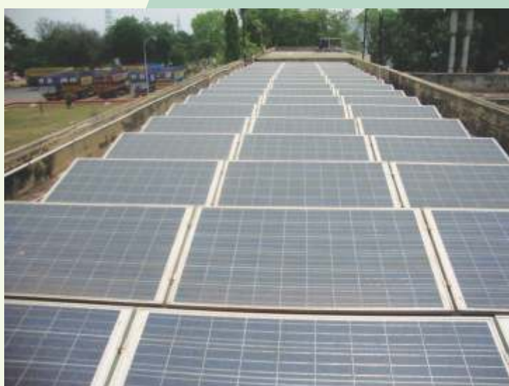
Solar panel - Pipeline, Chennai
