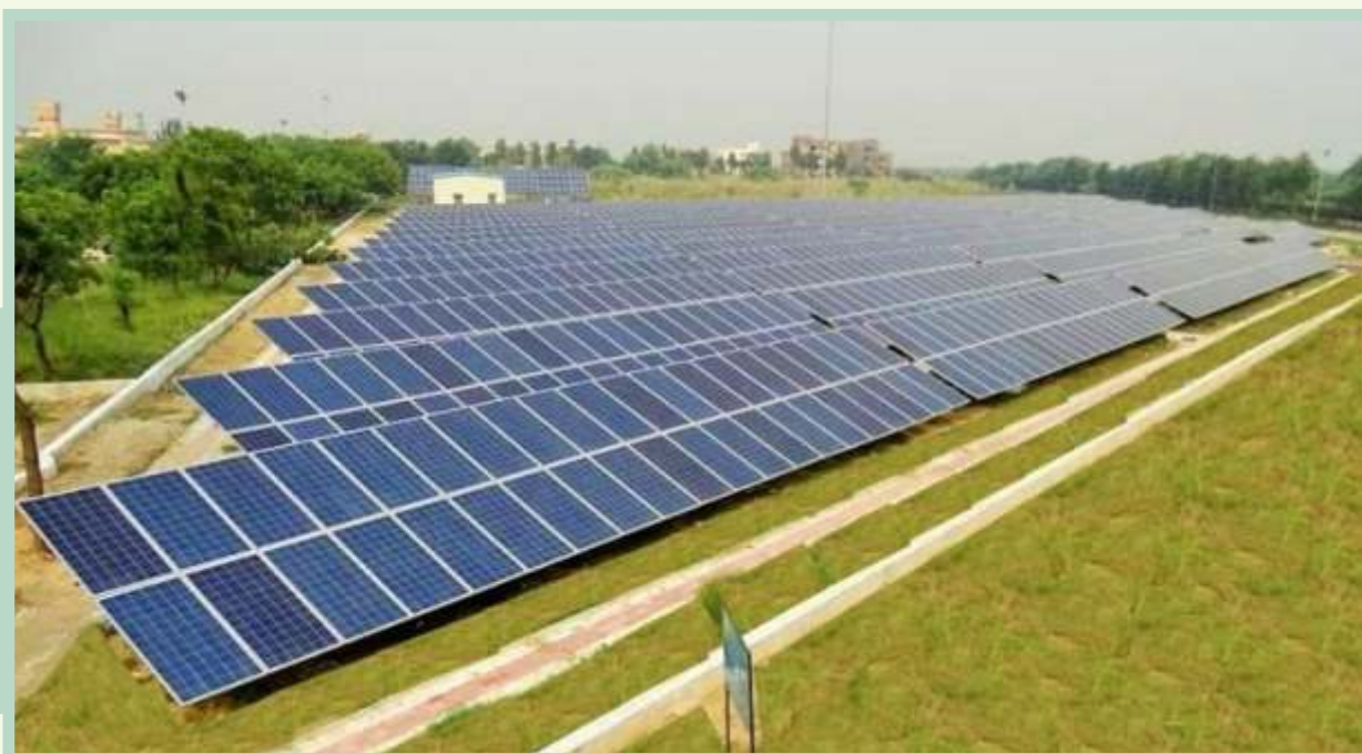
Photovoltaic Solar Module Array at Mumbai Refinery
