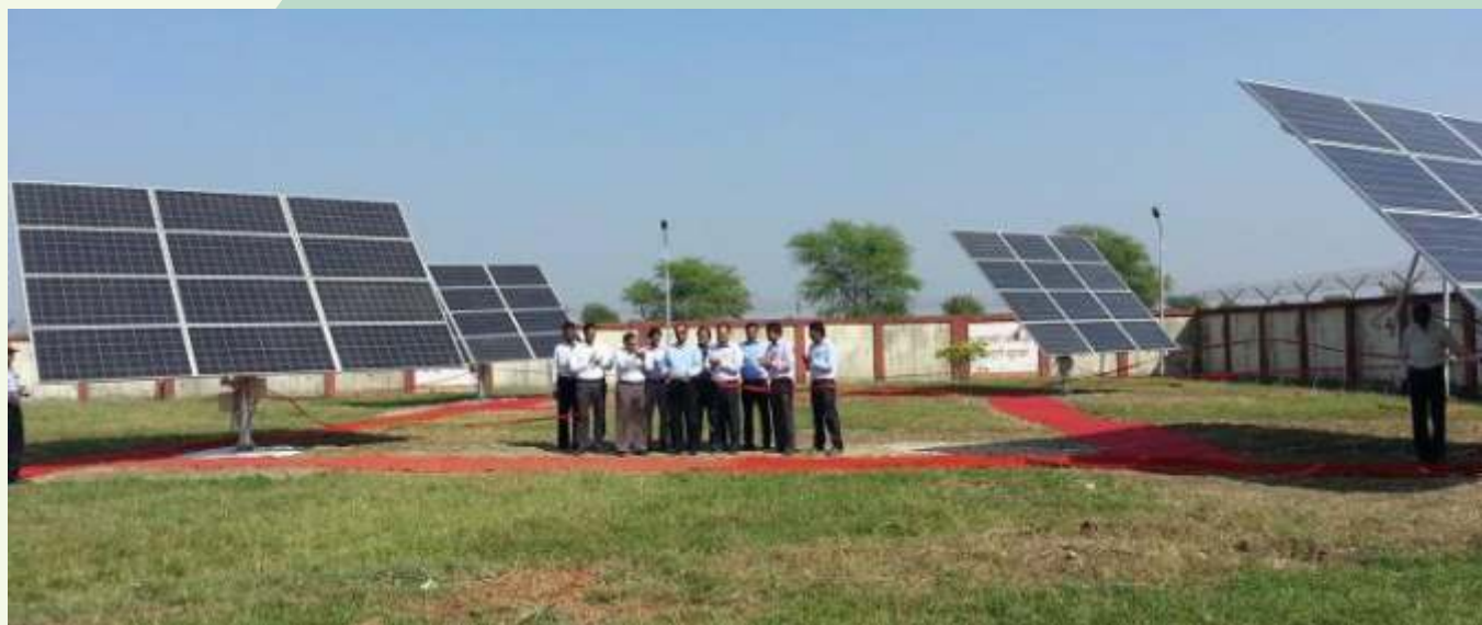
Alternate Source of Energy installation at Mumbai Refinery
