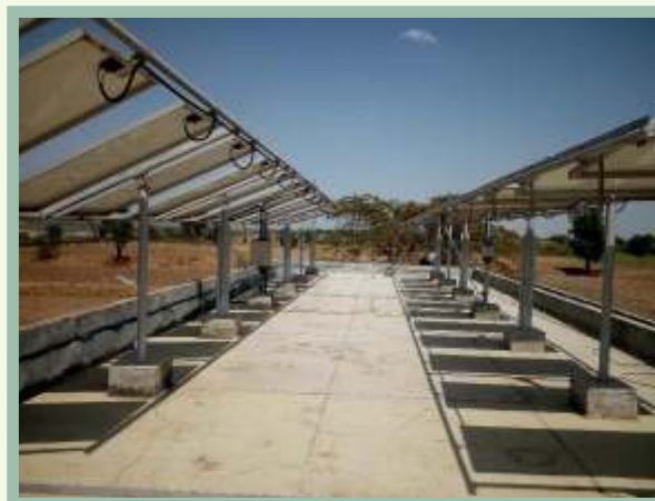
Solar Panels installed at the Pipelines - Chennai
